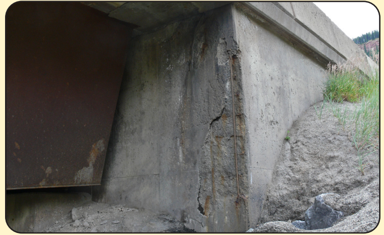
Image 6. Exposed rebar and Deteriorating Concrete on I-70 EBND over Polk Creek (F-12-AS)
